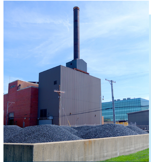
Mounds of coal awaiting use sit outside of the Capitol Power Plant, located in a residential area in Springfield.
